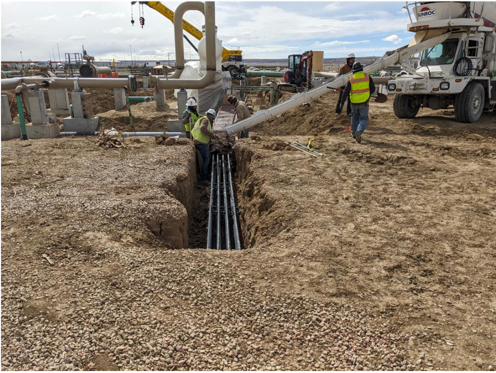
Location: Wamsutter Compressor Station Direction of Photo: N/A Description: Pouring red cement on the ducts. Date: 3/14/2025
