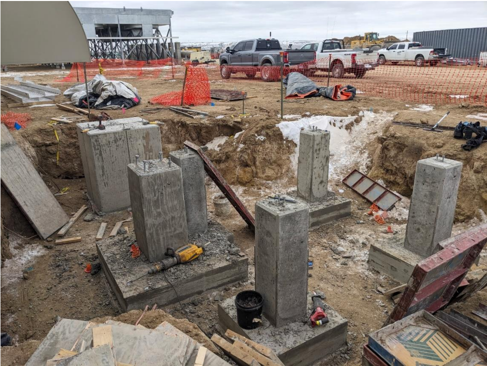
Location: Wamsutter Compressor Station Direction of Photo: N/A Description: Forms removed from the exhaust supports. Date: 2/19/2025
