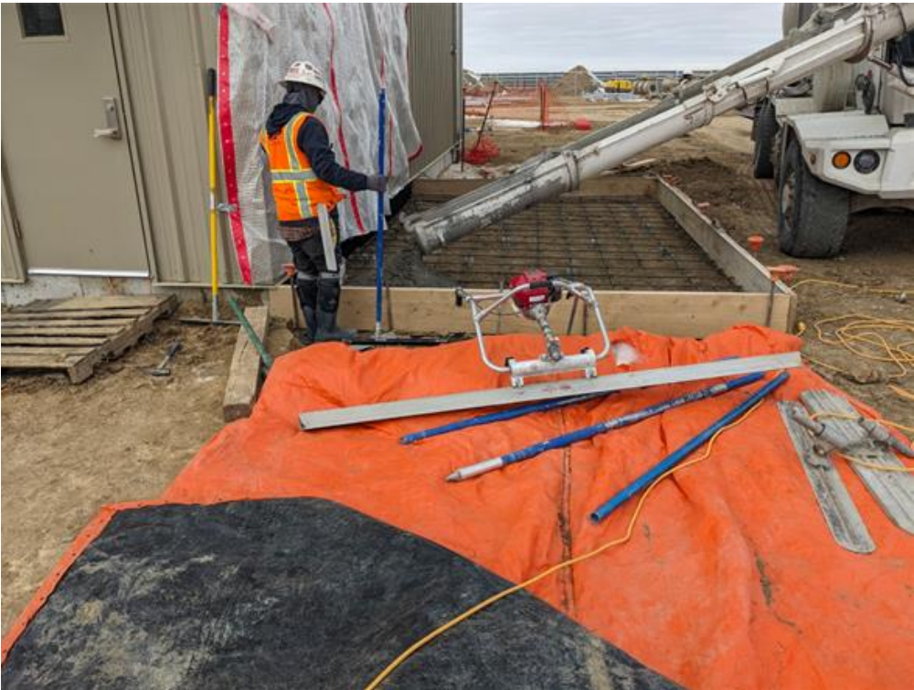
Location: Wamsutter Compressor Station Direction of Photo: N/A Description: Pouring concrete for the HVAC slab. Date: 2/19/2025
