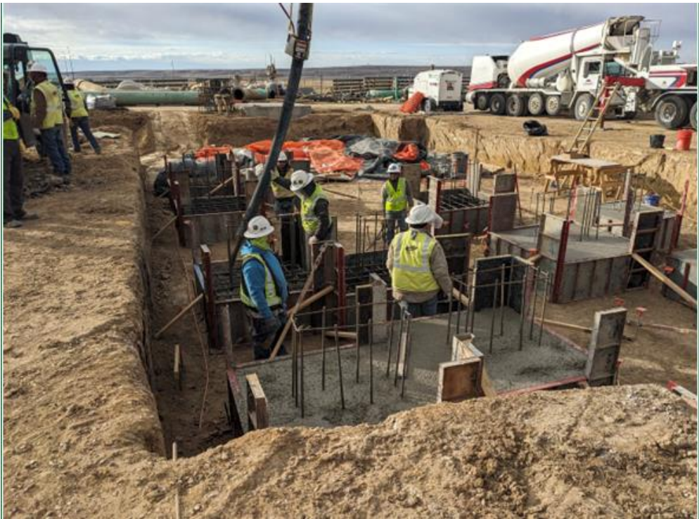
Location: Wamsutter Compressor Station Direction of Photo: N/A Description: Pouring concrete for the station recycle valve supports. Date: 2/07/2025
