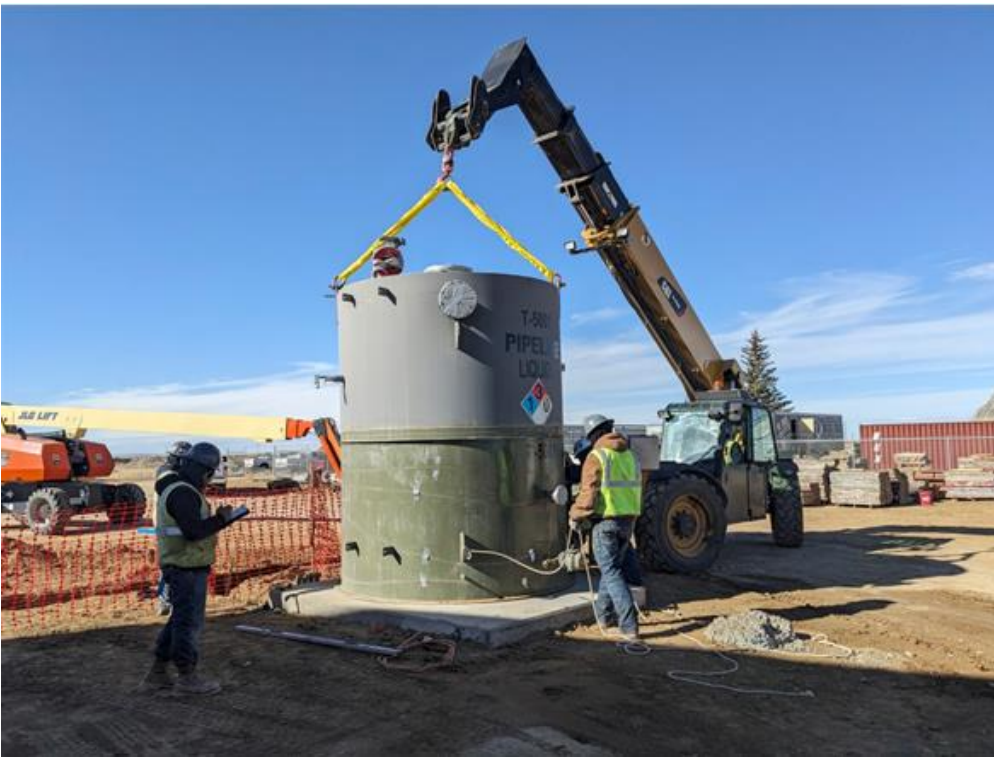
Location: Wamsutter Compressor Station Direction of Photo: N/A Description: Setting the wastewater tank on its foundation. Date: 2/06/2025
